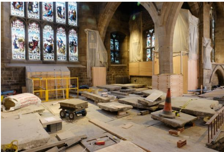
A jigsaw puzzle of old and new materials including bump protection coverings to at-risk areas.
